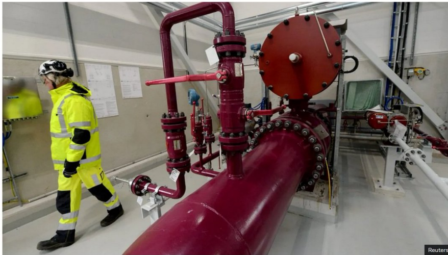
The Baltic-connector gas pipeline opened in 2020 and is used by both Finland and Estonia
