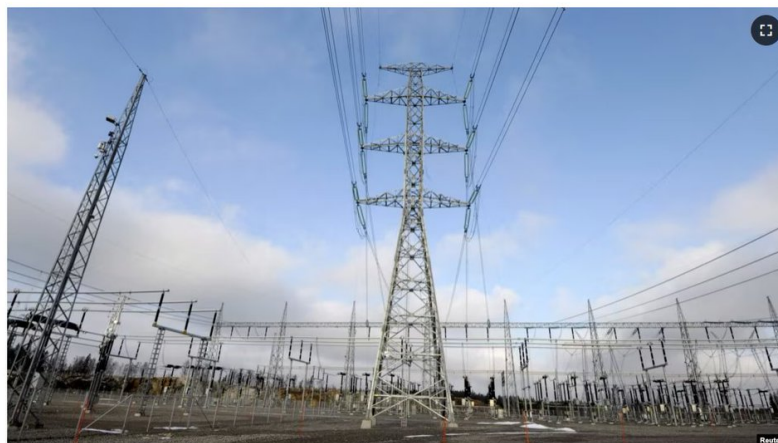
FILE - Fingrid's EstLink 2 transformer station operating between Finland and Estonia is pictured in Porvoo, Finland, March 6, 2014. Fingrid said current on the EstLink 2 cable was cut at 12:26 p.m. local time on Dec. 25, 2024. (Lehtikuija via Reuters)
