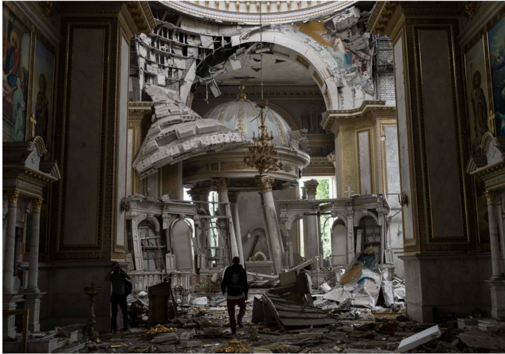
Church personnel inspect damages inside the Odesa Transfiguration Cathedral. Jae C. Hong/AP
